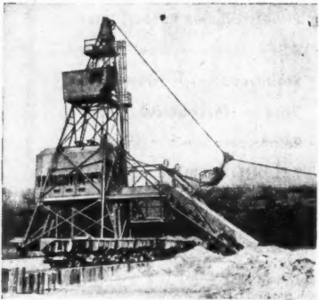
Mobile Sauerman Scraper unit loads material from open pit into cars at rate of 370 tons an hour.
